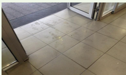
Figure 1.4: Showing slippery floor
